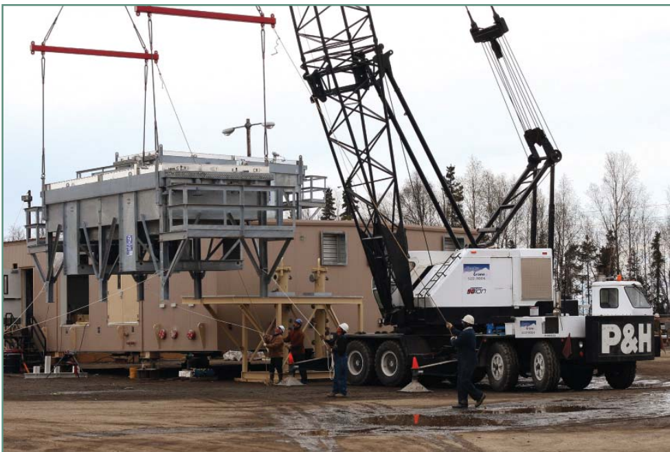
This photograph was taken at the AES Anchorage Fabrication Facility in May 2007. It shows a gas cooler being test fitted to roof of the Pioneer Natural Resources Oooguruk onshore gas compressor modules.
