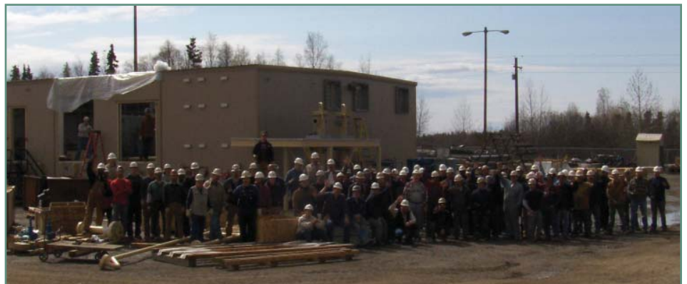
The crew at the AES Anchorage Fabrication Facility has been hard at work on the Pioneer Natural Resources Ooguruk module assembly project. This photograph, taken in May 2007, shows the crew in front of the onshore gas compressor modules as this successful year-long project nears completion.
